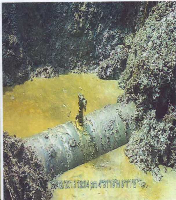
FIG 2: Spill point on excavation
